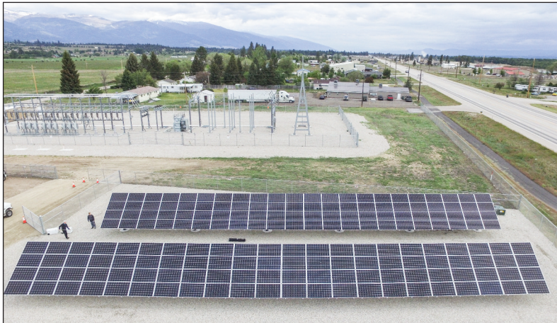
Aerial photo of Ravalli County Electric Cooperative's community solar project called Solar Valley. Courtesy of Ravalli County Electric Cooperative
