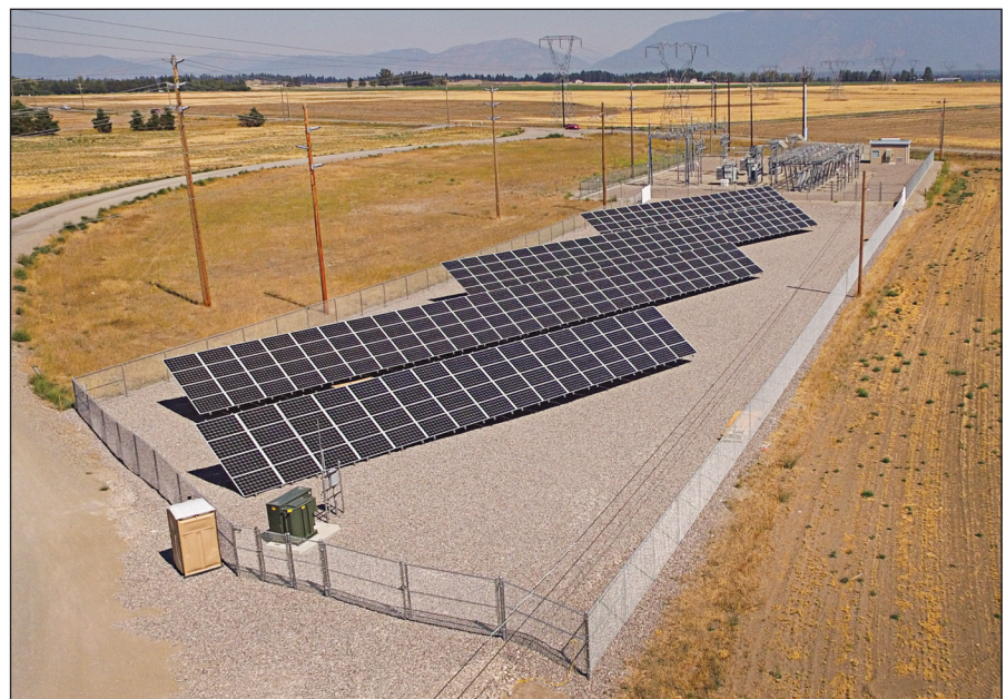
Photo by Mike Radel, Flathead Electric Cooperative
