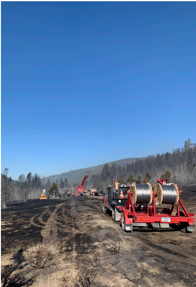
VEC line crew rebuild power line in the aftermath of the Deep Creek Fire. | VEC FILE PHOTO
