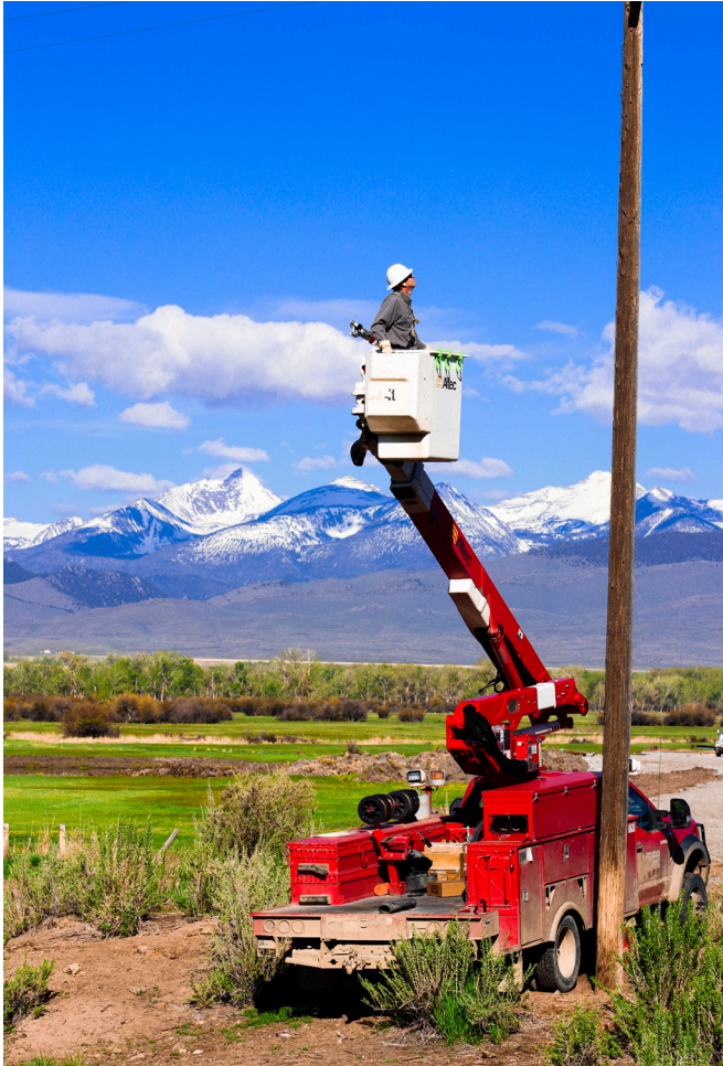
Lineman Tyler Arnio is preparing to lift a power line to create enough clearance for a house that was being relocated. | PHOTO TAKEN BY PAIGE GARRISON
