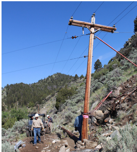
Pictured is a pole that our line crew replaced where we had to shut down the power in order to replace the pole safely.
