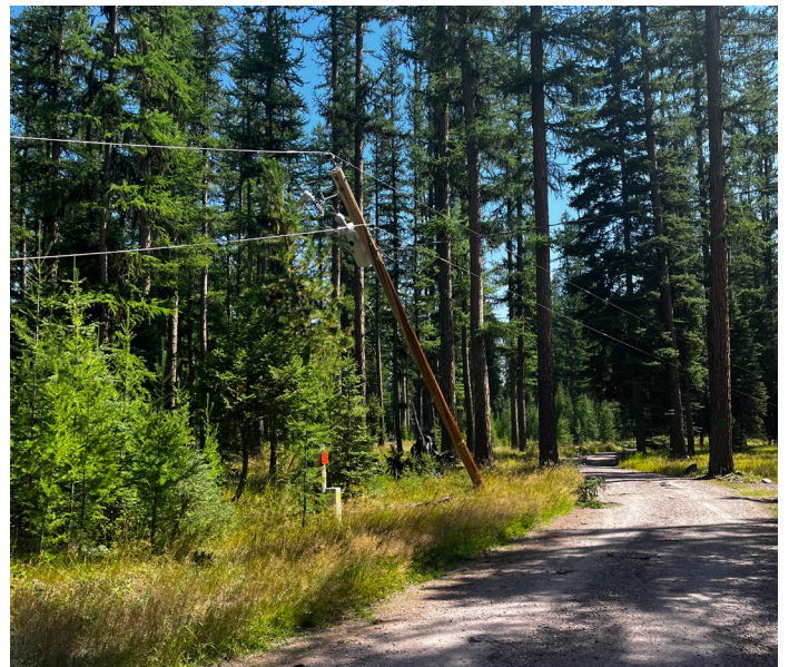
Pictured is storm damage sustained in Missoula Electric Cooperative's service territory. This was one of two storms this past summer in which Vigilante Electric linemen assisted in power restoration efforts.
